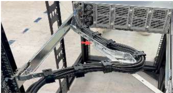
CMA installed on JBOD.
